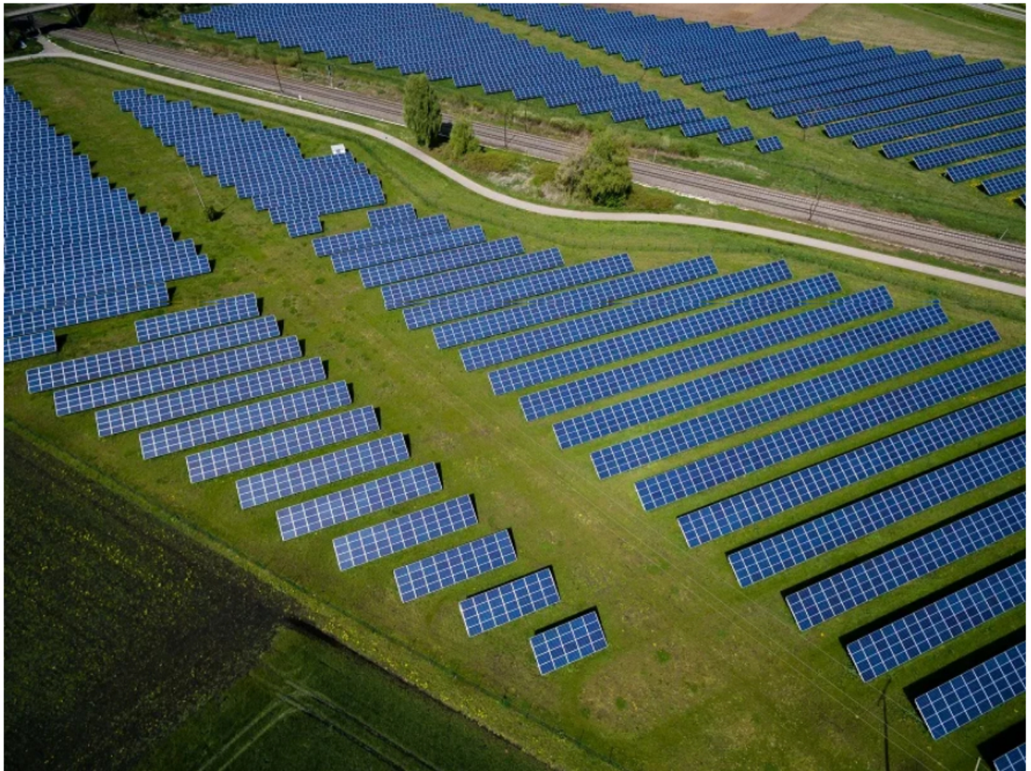
The solar project will feature 180,000 monocrystalline bifacial panels. Credit: Andreas Gückhorn / Unsplash.
